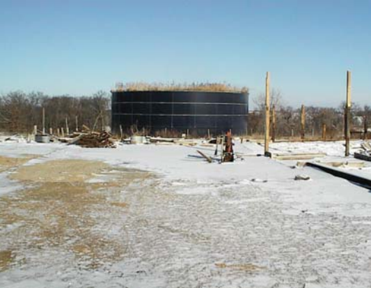
Pre-Qualified Slurry Store Structure
